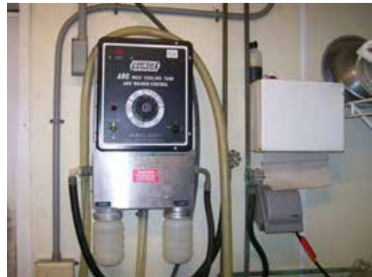
The control panel for the bulk tank has a constant temperature reading of the temperature of the milk in the bulk tank and runs the automatic wash system for the bulk tank.
