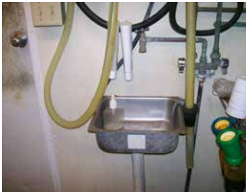
A separate sink should be available for washing hands of the milkers. The two sinks used for washing and sanitizing equipment may not be used for this purpose.
